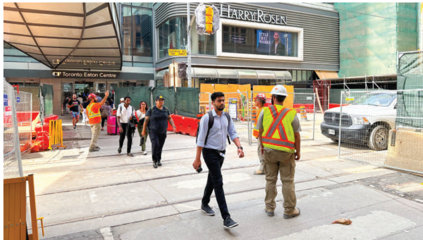
DESPITE BEING CLOSED TO VEHICULAR TRAFFIC FOR SUBWAY STATION CONSTRUCTION, PEDESTRIAN TRAFFIC REMAINS HIGH ON QUEEN STREET.
