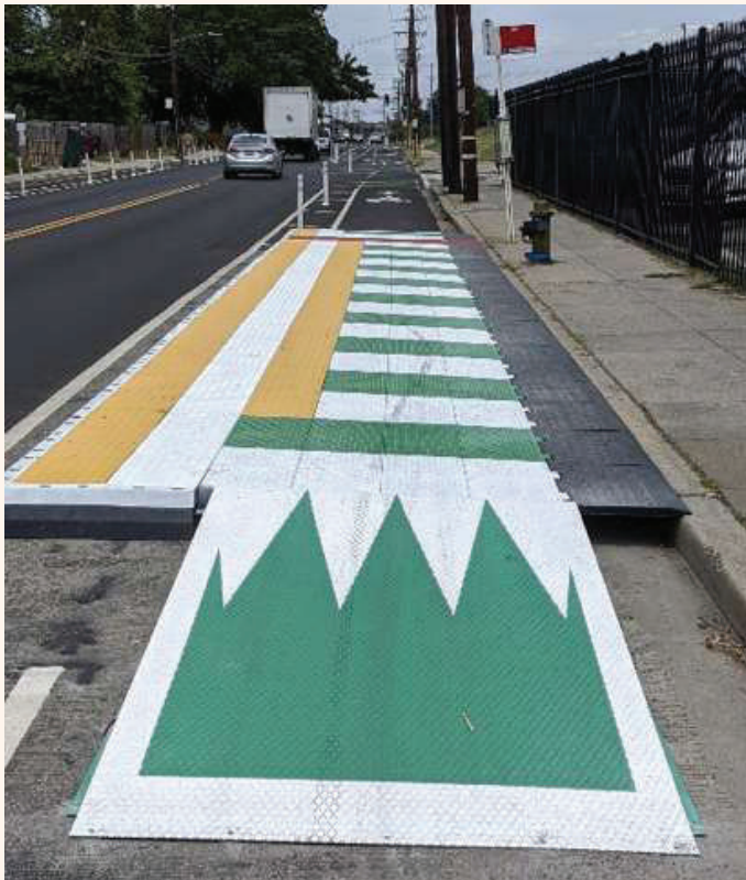
WASHINGTON, DC HAS INSTALLED PLASTIC LOADING PLATFORMS THAT ARE USED UNTIL THEY CAN BE REPLACED BY PERMANENT CONCRETE INSTALLATIONS.
